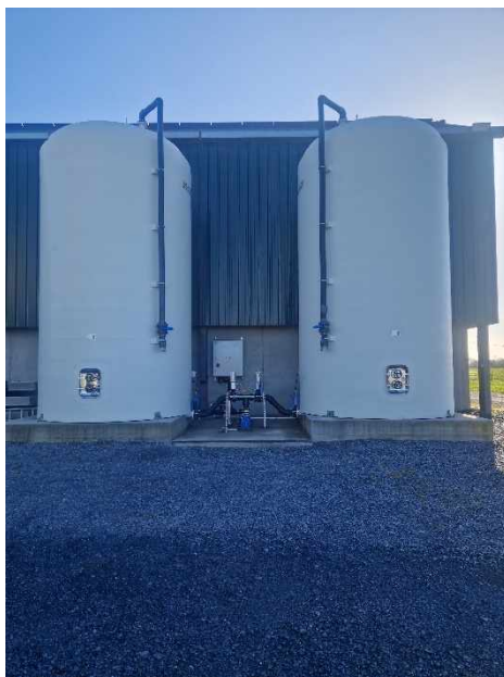
Cuves de stockage de glycérine BIOMETHABEARN 2024
